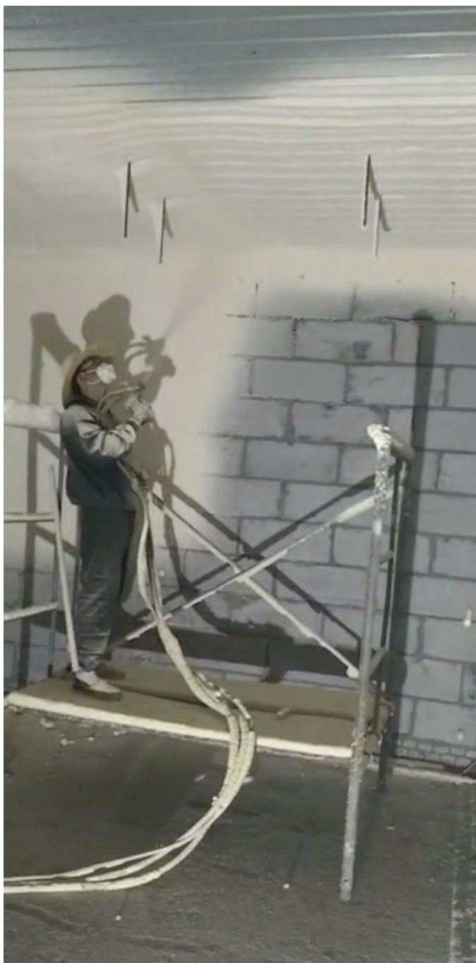
Dacheng Wan Fu Chemical Co. Ltd spraying foam in a cold storage warehouse in Hebei Province, China.
