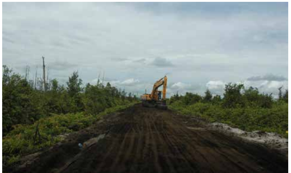
Figure 15 Road compaction work in Marang by Palangkaraya Municipal Public Works and Spatial Planning Agency using heavy machinery (December 2016)
