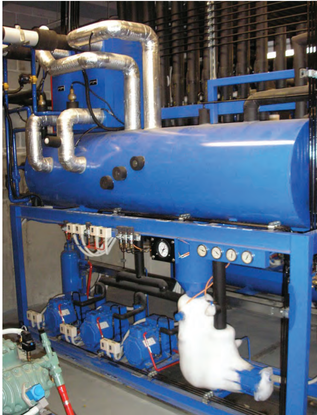
CO 2 sub-critical supermarket cascade refrigeration system
