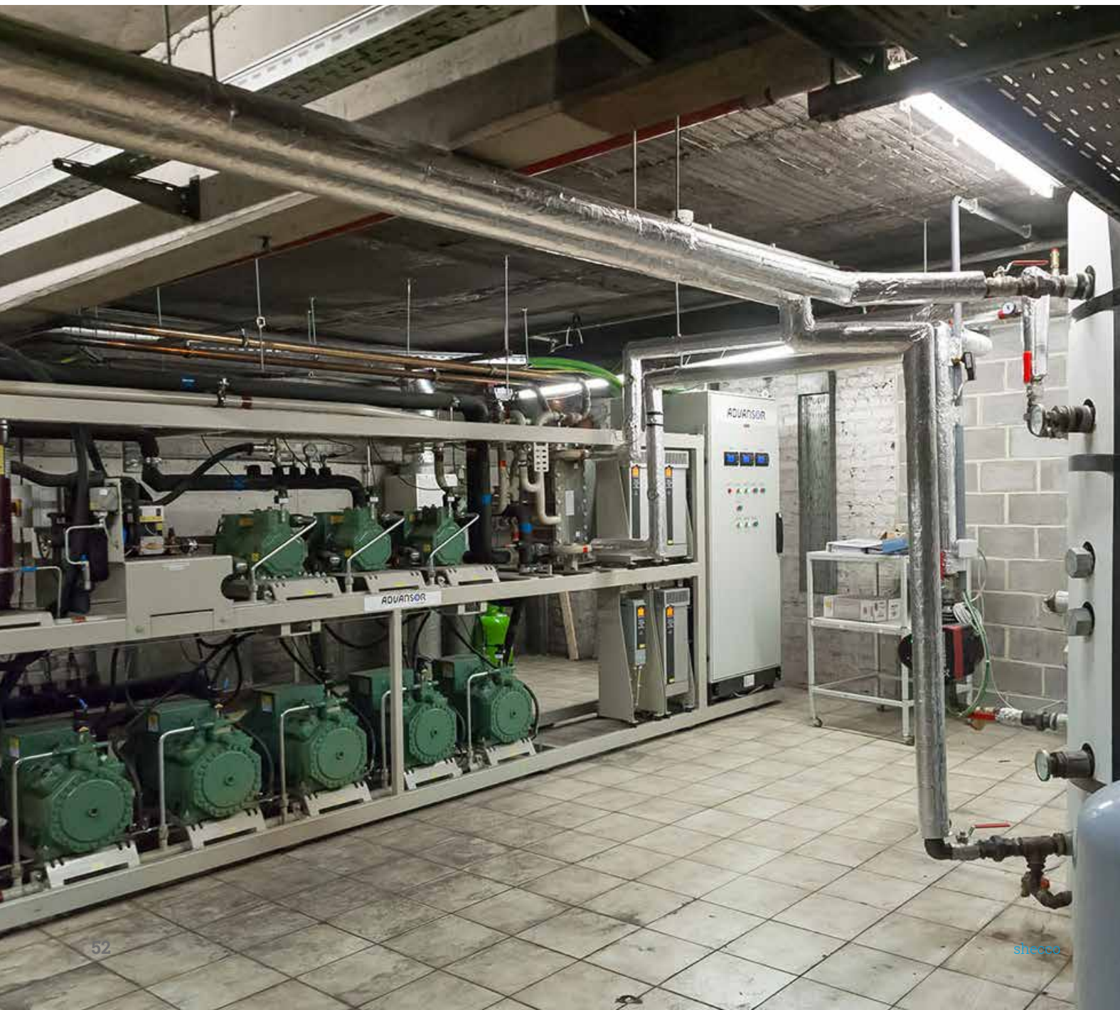
Below: CO 2 transcritical rack with heat reclaim used at a Delhaize supermarket in Belgium
