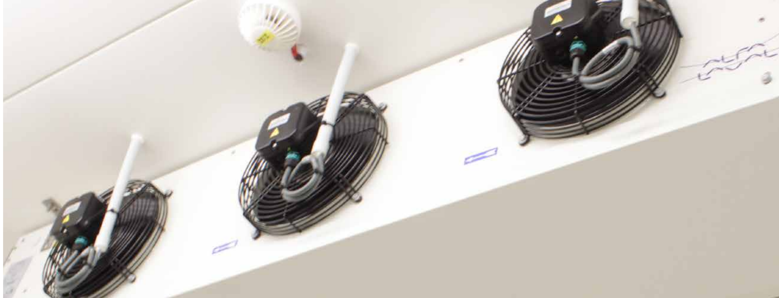
Above: Alfa Laval fans in a biostore
