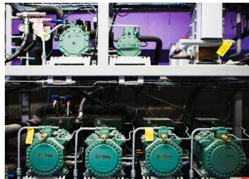
Compressors on a CO 2 transcritical rack
