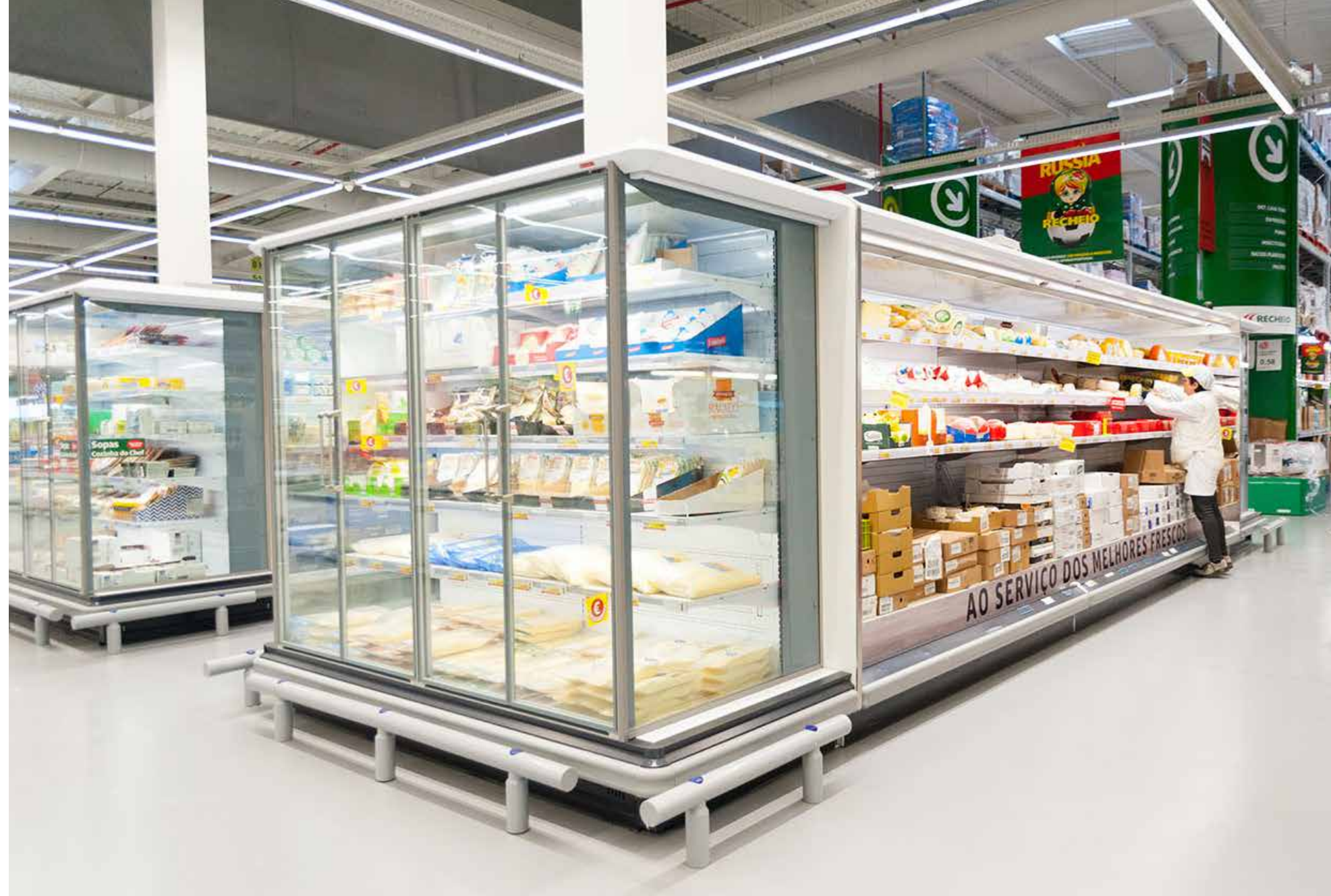
Above: Recheio Cash & Carry in Portugal using a CO 2 transcritical with heat reclaim system
