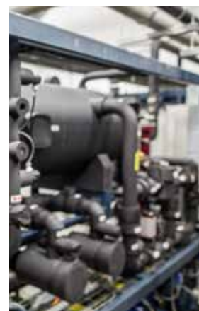
Equipment shot of a CO 2 transcritical rack
