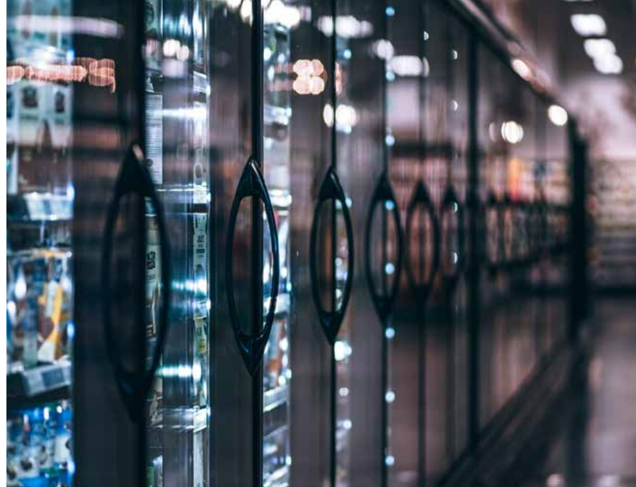
Above: A supermarket at night with lights in display cabinets left on
