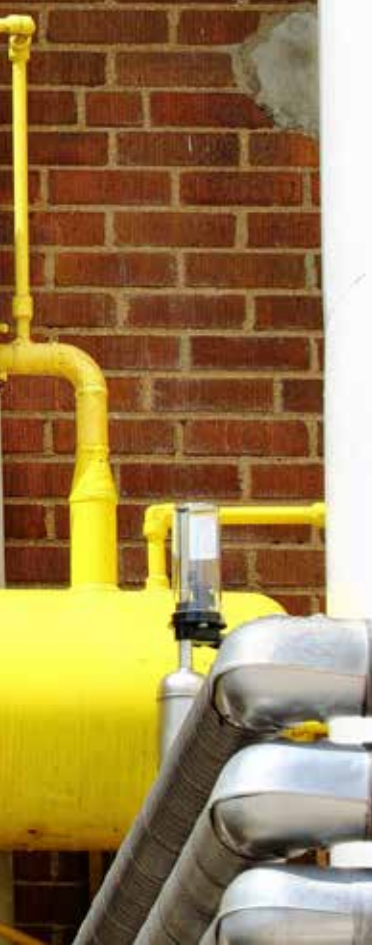
Above: Ammonia refrigeration piping and tanks
