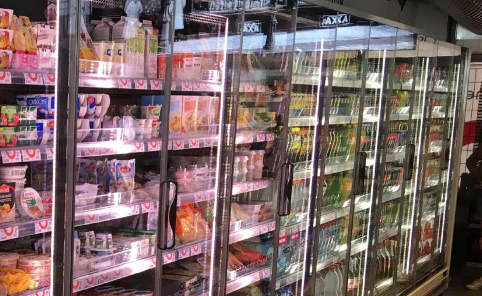
Above: Refrigerated display units with doors and LEDs
