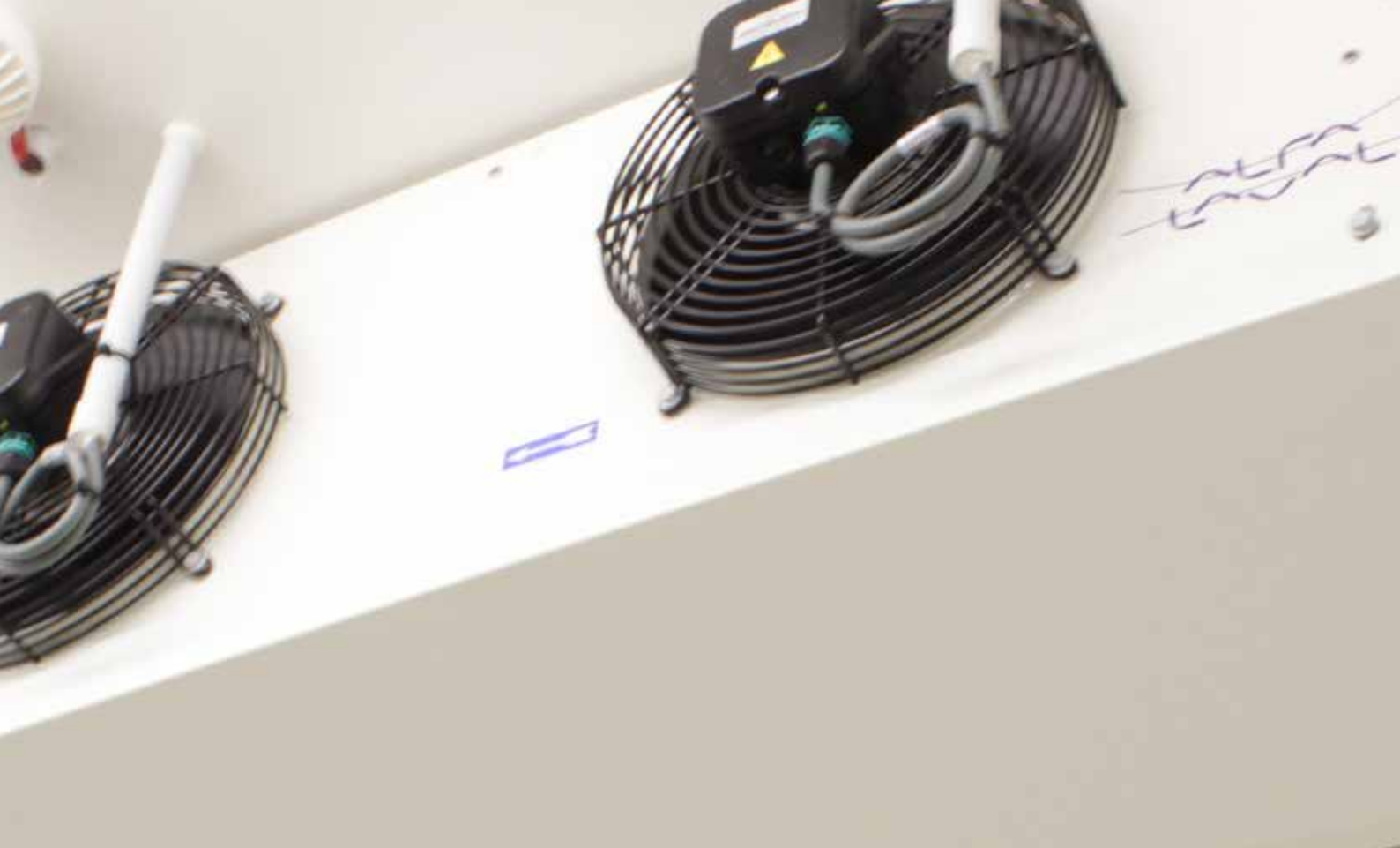
Above: Alfa Laval fans in a biostore
