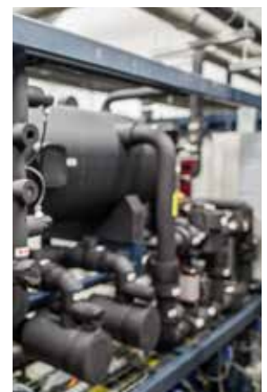
Equipment shot of a CO 2 transcritical rack
