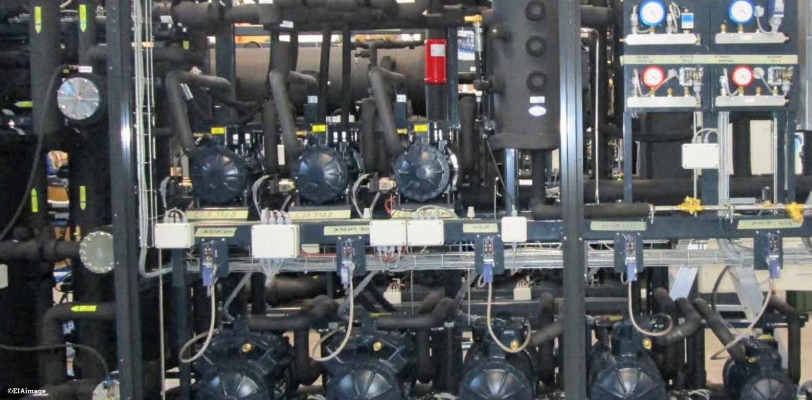
Above: CO 2 transcritical rack in Al-Salam supermarket in Jordan
