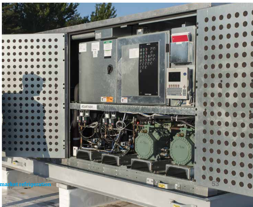
Below: CO 2 transcritical rack used at an ALDI US store in New York
