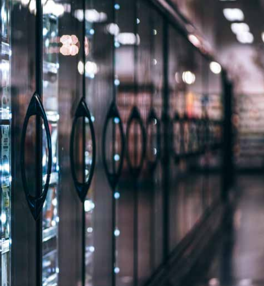
Above: A supermarket at night with lights in display cabinets left on
