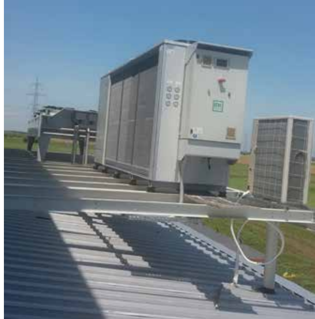
Mechanical sub-cooler with HC-290 for a CO 2 transcritical system in Romania
