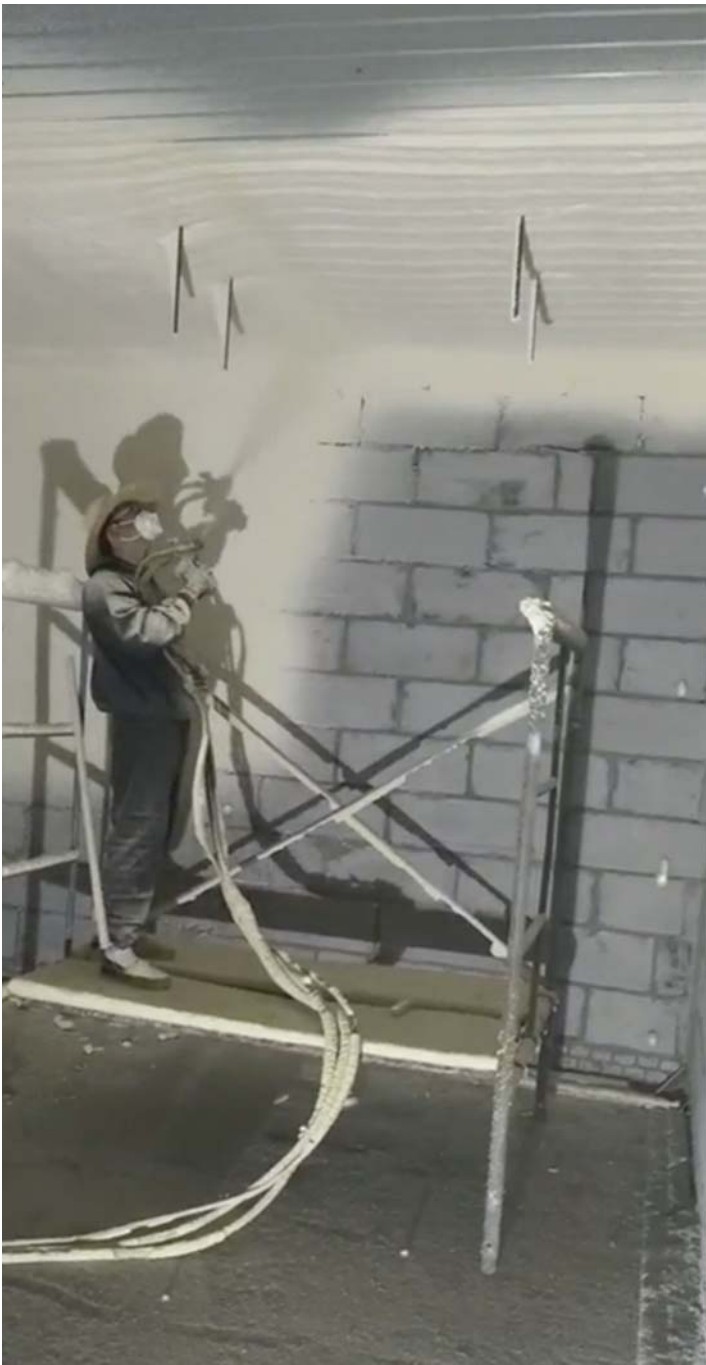
Team from Dacheng Wan Fu Chemical Co. Ltd spraying foam in a cold storage warehouse in Hebei Province, China
