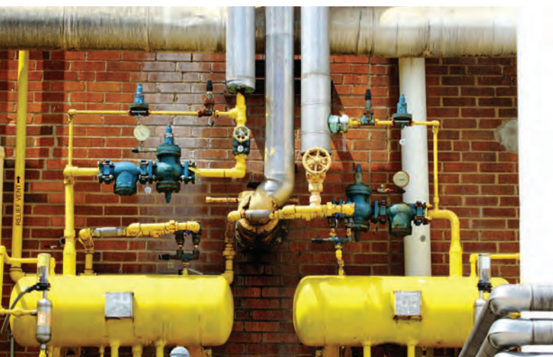
Above: Ammonia refrigeration tanks.
