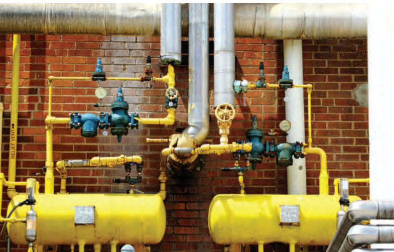
Above: Ammonia refrigeration tanks.
